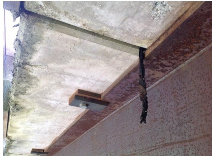
rubber seals rotted out
